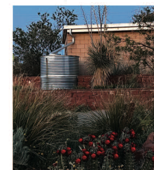
Whitfield's rain harvesting system brings water through gutters and downspouts to a galvanized steel cistern. A connecting hose conveys water to native plants. Photo by Teresa Smith de Cherif.
